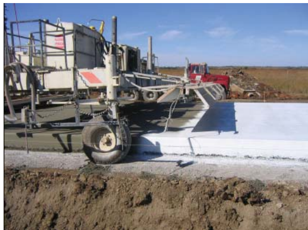
Figure 6. Uniform application of curing compound to slab surface and sides (Taylor et al. 2006)
