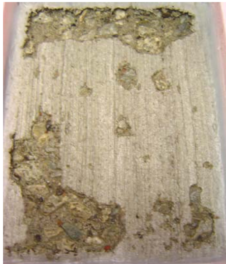
Figure 2. Concrete scaling caused by deicing chemicals (Sutter 2008)
