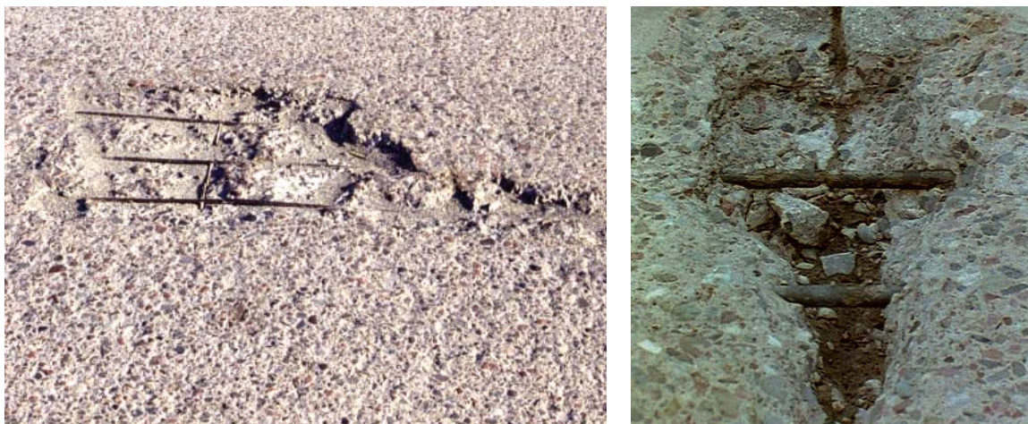
Figure 3. Corrosion of high steel (left photo) and of embedded dowel bars (right photo)
