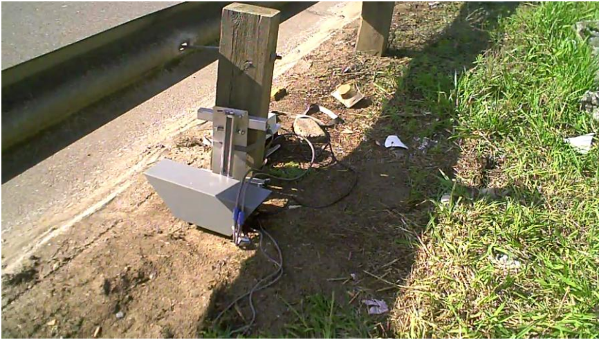
AxleLight mounted to guard rail at TH 52 Test Site.
