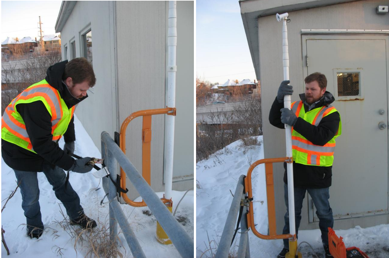
Figure 34. Miovision Setup at NIT Test Site (Railing Mount)
