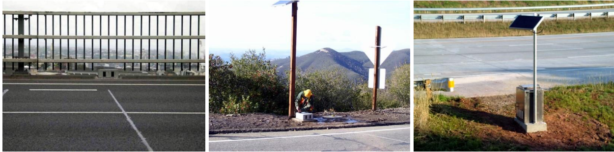
Figure 29. Roadside/Pad-Mounted TIRTL Sensors (Permanent Installation)
