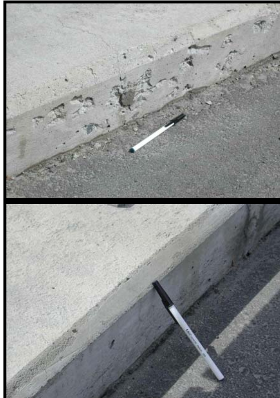
Phase I: West Lebanon bridge repair after two winters. Top = control concrete noticeably spalled. Bottom = antifreeze concrete in good condition. Phase II testing corroborates this result by suggesting that antifreeze concrete can be more durable than ordinary concrete.
