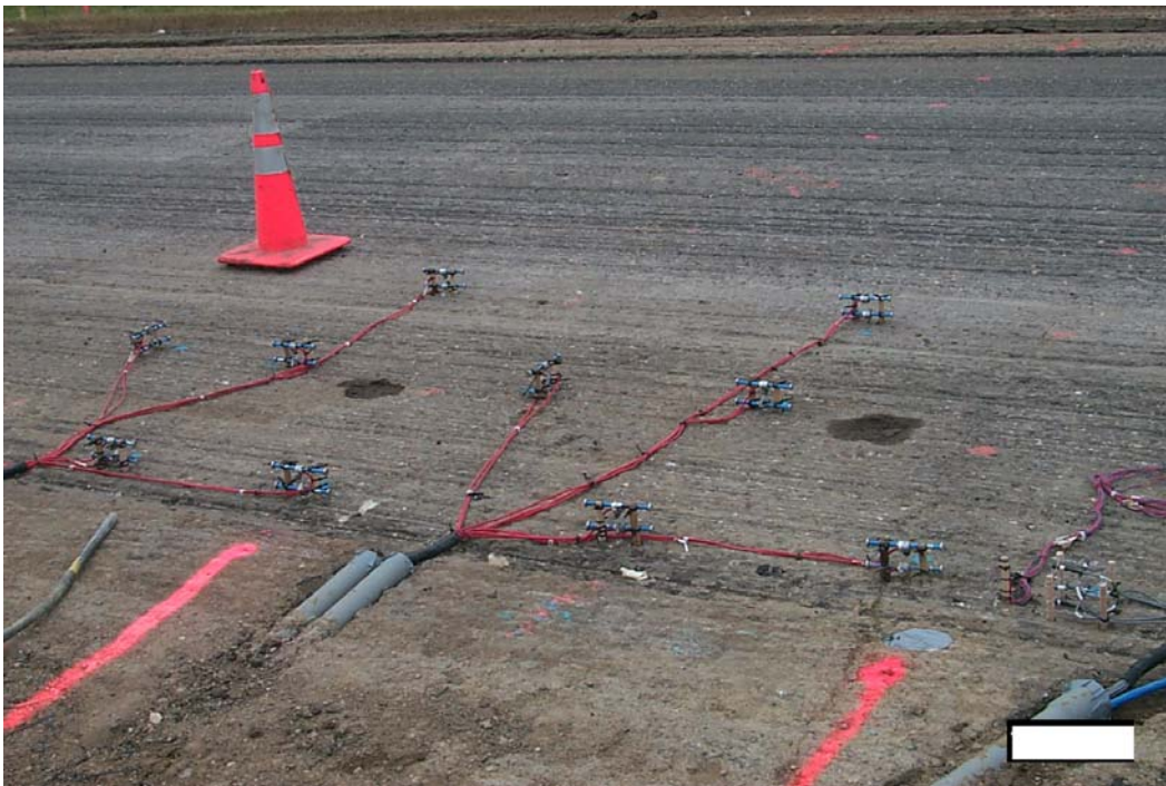
Photo 2: Installation of sensors in new MnROAD thin-whitetopping cells, October 2004. The sophisticated set up of instrumentation in the whitetopping sections at MnROAD, provides valuable field data that can be used in the development of a whitetopping design method.
