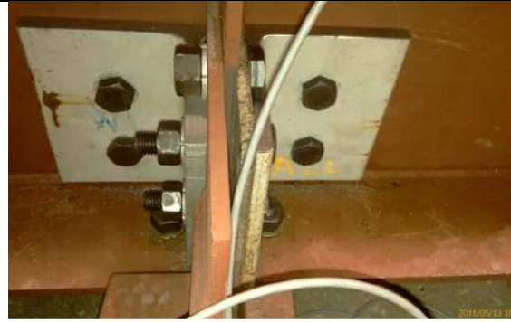
Fig. 4 View of angles bolted to the connection stiffener and girder web on the interior of Specimen 3
