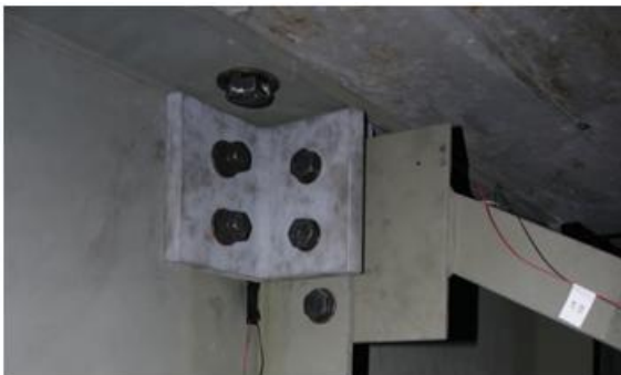
Figure 1. View of double angles and backing plate retrofit on interior face of an exterior girder.
