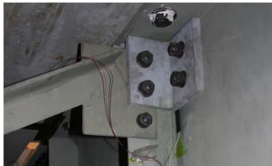
Figure 2. View of double angles and backing plate retrofit on interior face of an exterior girder.
