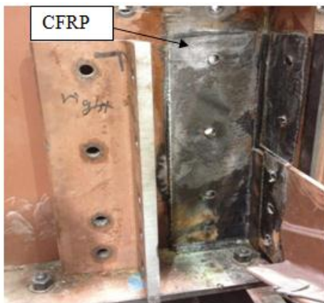
Figure 6. View of the steel-CFRP sandwich retrofit applied to Specimen 3 (interior face of girder; left side of connection stiffener) – steel angle has been removed from the CFRP in this view
