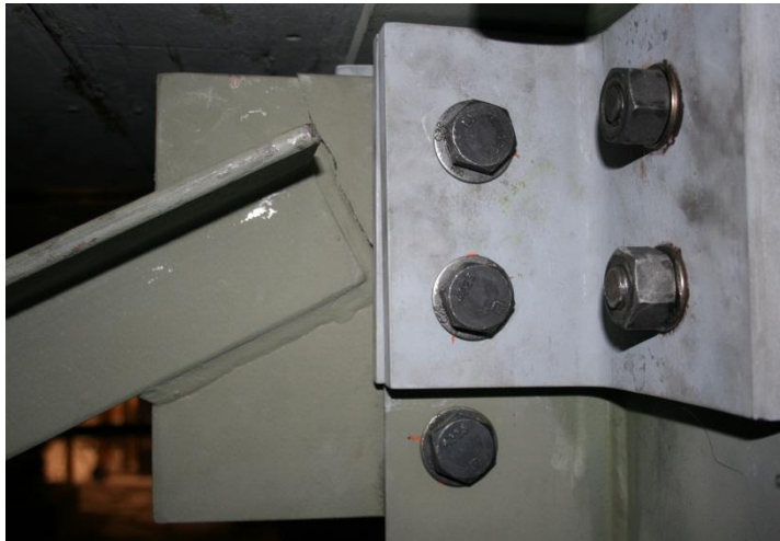
Figure 4. View of crack in the cross frame table plate before removal of the cross frame
