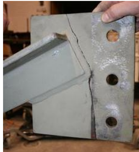
Figure 5. View of cracked tab plate after cross frame removal
