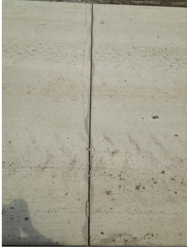
Figure 6. Crack at Site 2
