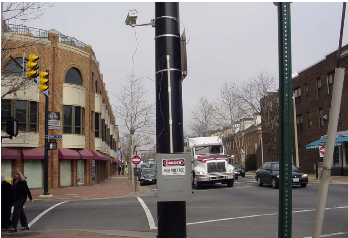
Figure 6. The PATH video recording system installed at the control site
