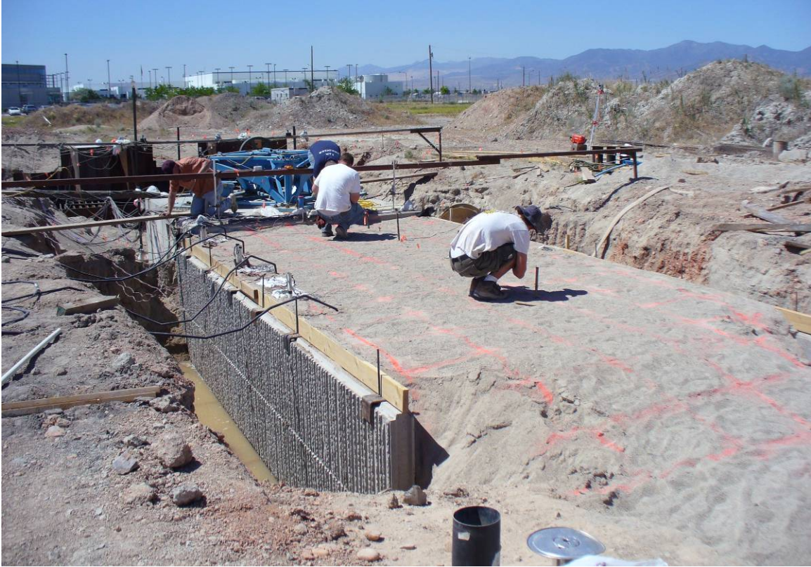
Fig 2. Dense sand backfill compacted between two MSE walls which are flush with the outside edge of the 11 ft wide pile cap and extend 24 feet behind the pile cap.
