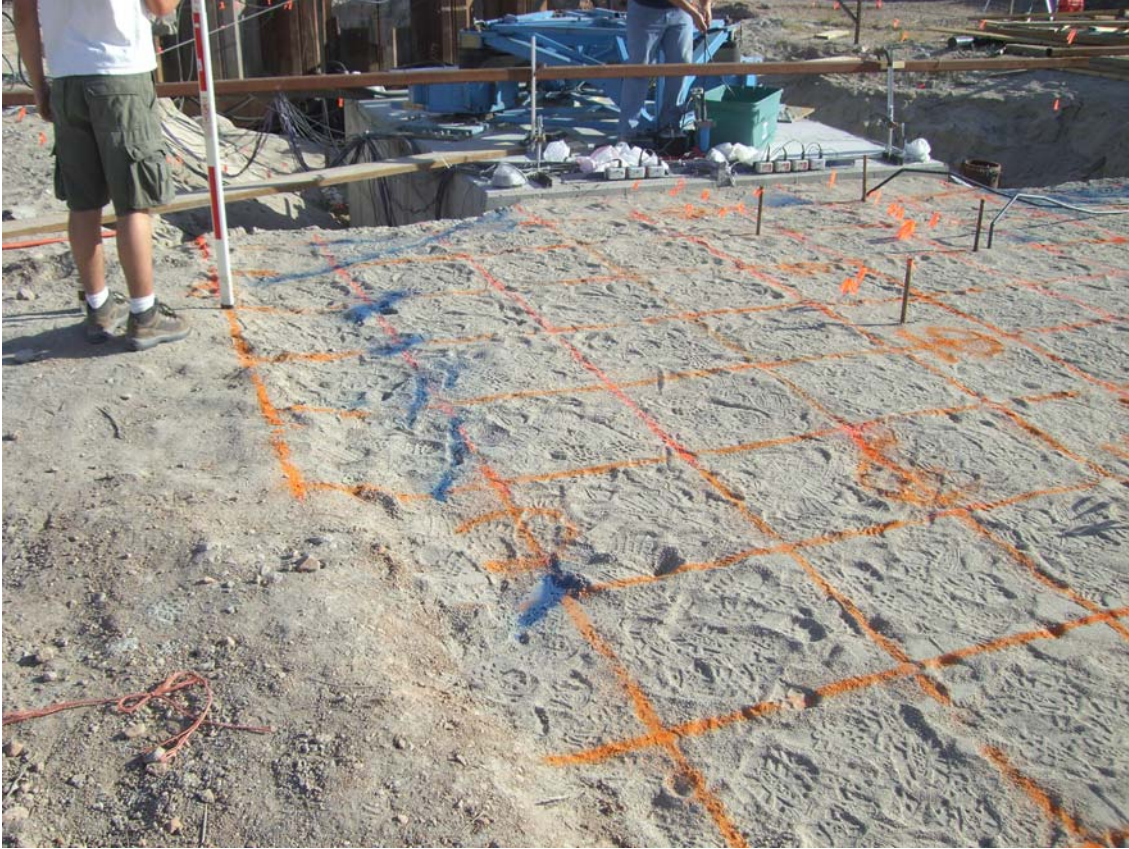
Fig. 1. Dense sand backfill extending about six feet beyond the edge of the pile cap on either side. Orange grid lines are 2 ft x 2 ft. Shear cracks are painted in blue and indicate an effective pile cap width of approximately 19.5 ft.
