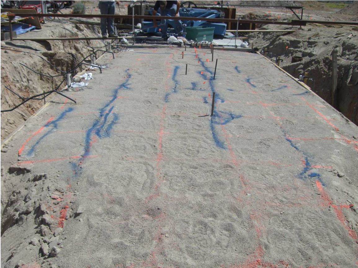
Fig. 4 Longitudinal cracking due to lateral displacement of the MSE wall during passive pressure testing.
