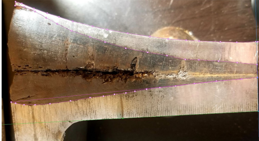
Figure 1 – Mapped corrosion for FE modeling from member obtained from Minnesota
